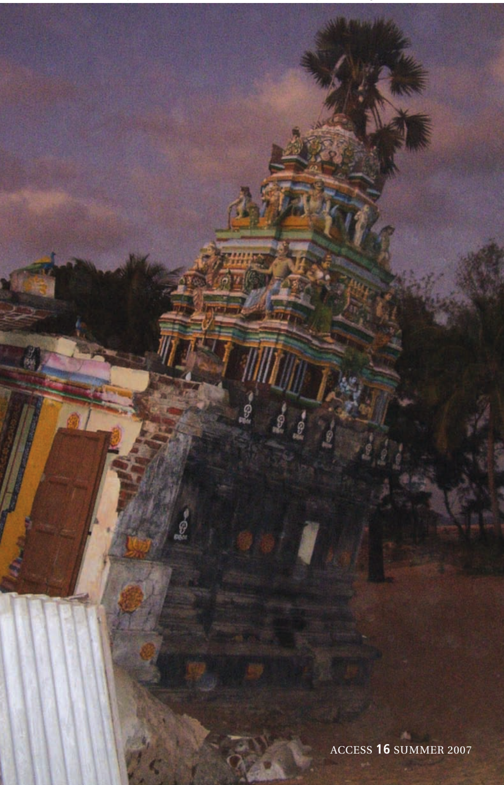
A Hindu temple in Batticaloa, Sri Lanka which collapsed during the tsunami.
